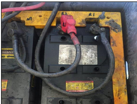
Image 3 – Failed battery in portable charging trolley
